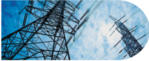
POWER TRANSMISSION & DISTRIBUTION
