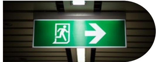
EMERGENCY AND SAFETY SYSTEMS
