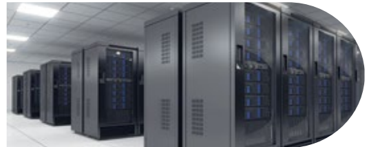
LARGE DATA CENTRE
